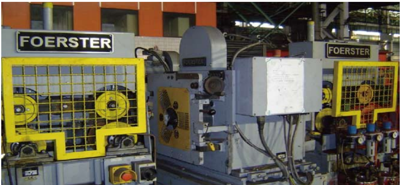
A、B、C、D线棒材漏磁探伤设备 magnetic flux leakage testing equipment for wire and bar installed in Line A, Line B, Line C and Line D
